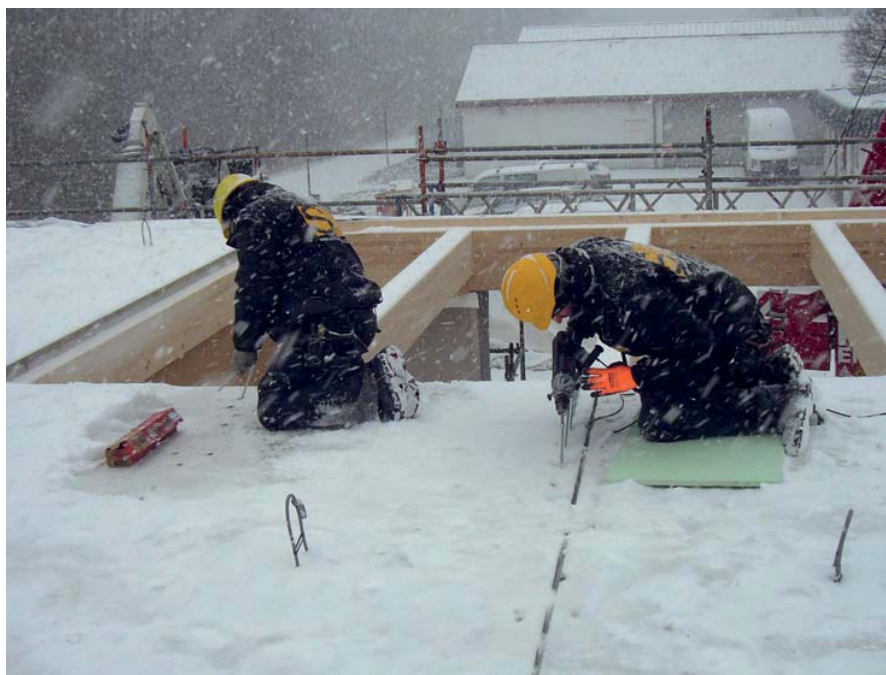
Installation of a finished product slab with finished product (FP) connectors even during winter conditions
