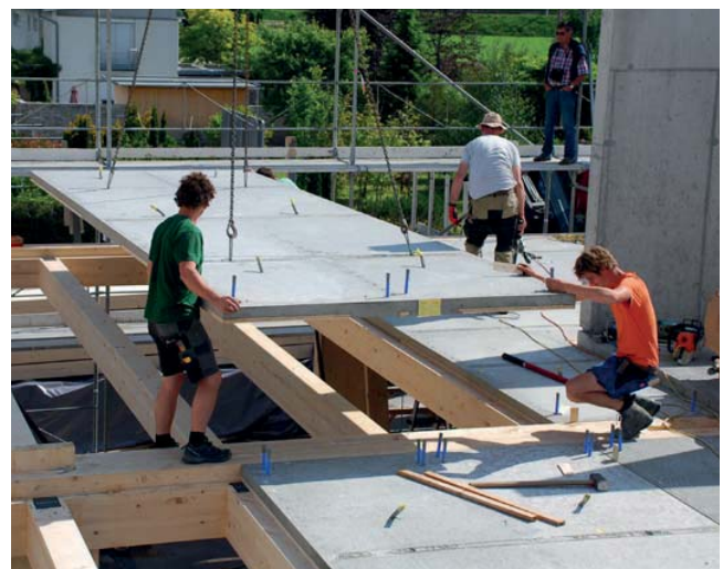
Installing pre-fabricated slabs with FP connectors on a layer of beams (here integrated mass activation for heating and cooling included)
